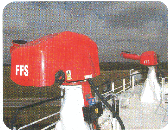
The foam monitors are located on top of the wheelhouse
